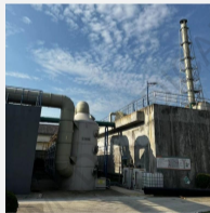
Sludge Drying and Deodorization facilities
